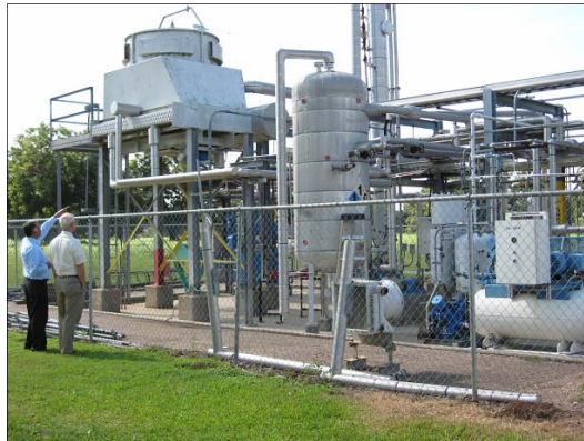
Pilot plant at Brazosport Community College in Texas, similar to plant being designed for BTC
